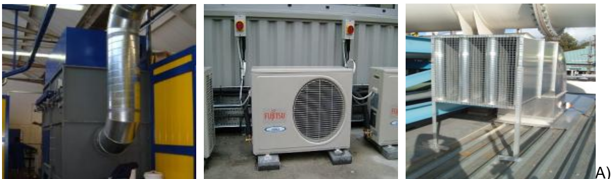
a) Dust extraction unit b) Air conditioning unit c) Roof extraction fan
