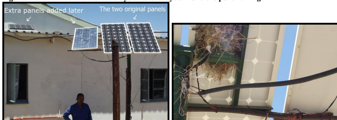
Figures 1 and 2: Mr. Titus and his dysfunctional system and the panel wiring
