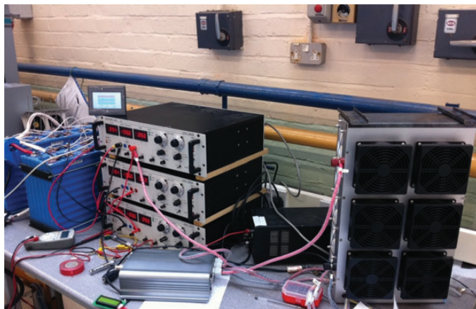
Figure 1. Configuration of the FCs and batteries hybrid system.
