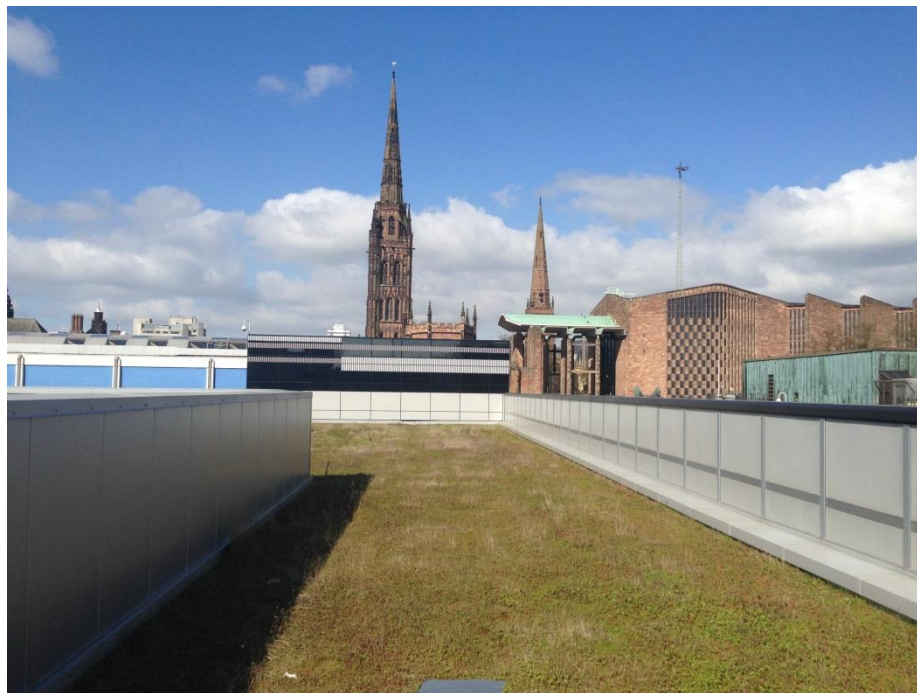
Figure 2-11 Green Roof on the Students Union at Coventry University.
