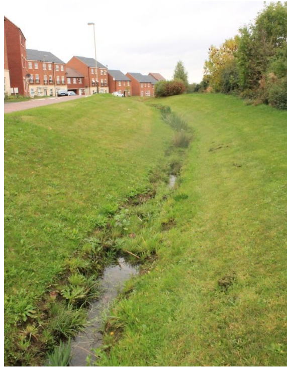
Figure 2-13 Swale at Hamilton SuDS Management Train, Leicester, that conveys runoff from detention basins and wetland areas.
